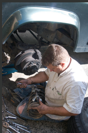
Above: Old spring out ready for a new spring and shock going in.
